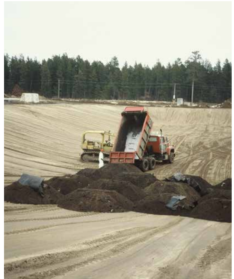
1986 : Contaminated soil being dumped into the containment vault (OU2), which has sand covering the initial plastic lining.
